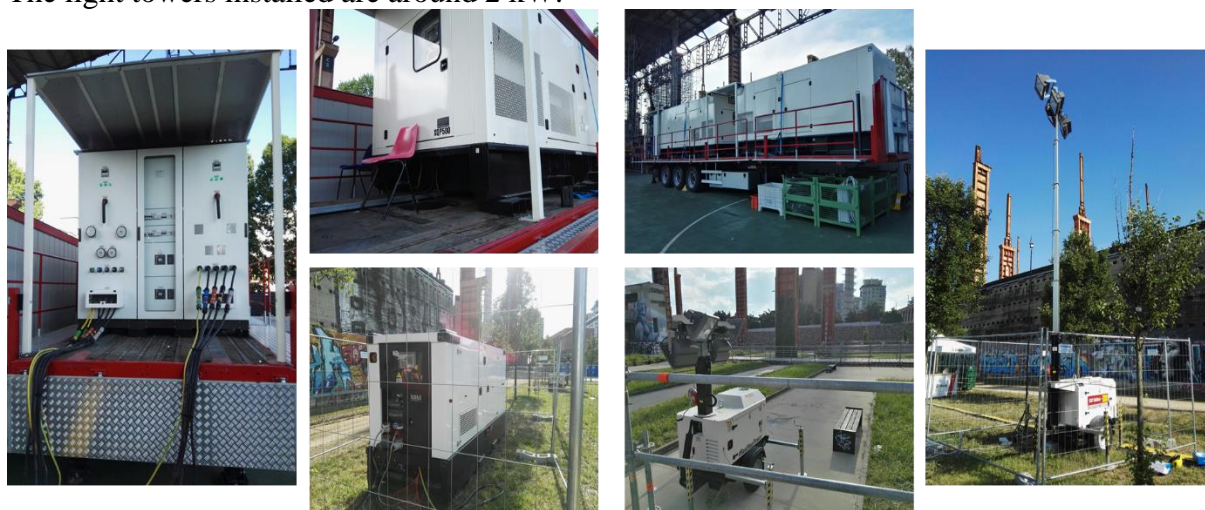
Figure 1. Gensets installation during the KappaFuturFestival (Turin_Parco Dora 6-7 July 2018).
